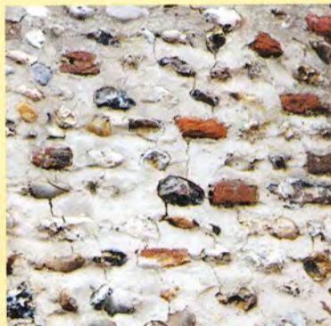
This crack pattern is typical of cement mortar pointing into flint. The pointing is no longer excluding water but trapping it, raising the moisture level within the wall
