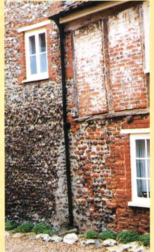
The downpipe has been repaired, but repairs to the wall with cement pointing will not last and form an ugly patch. Below the eaves, ancient lime wash is still evident with the brickwork substrate it once covered, completely undamaged.
