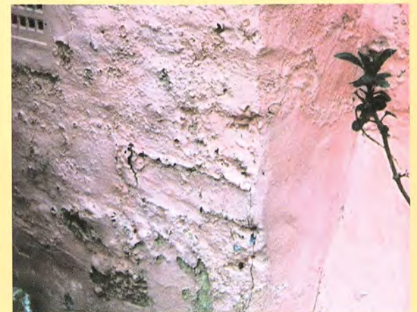
Without a DPC, the need to maintain vapour permeance to the external surface becomes critical.
